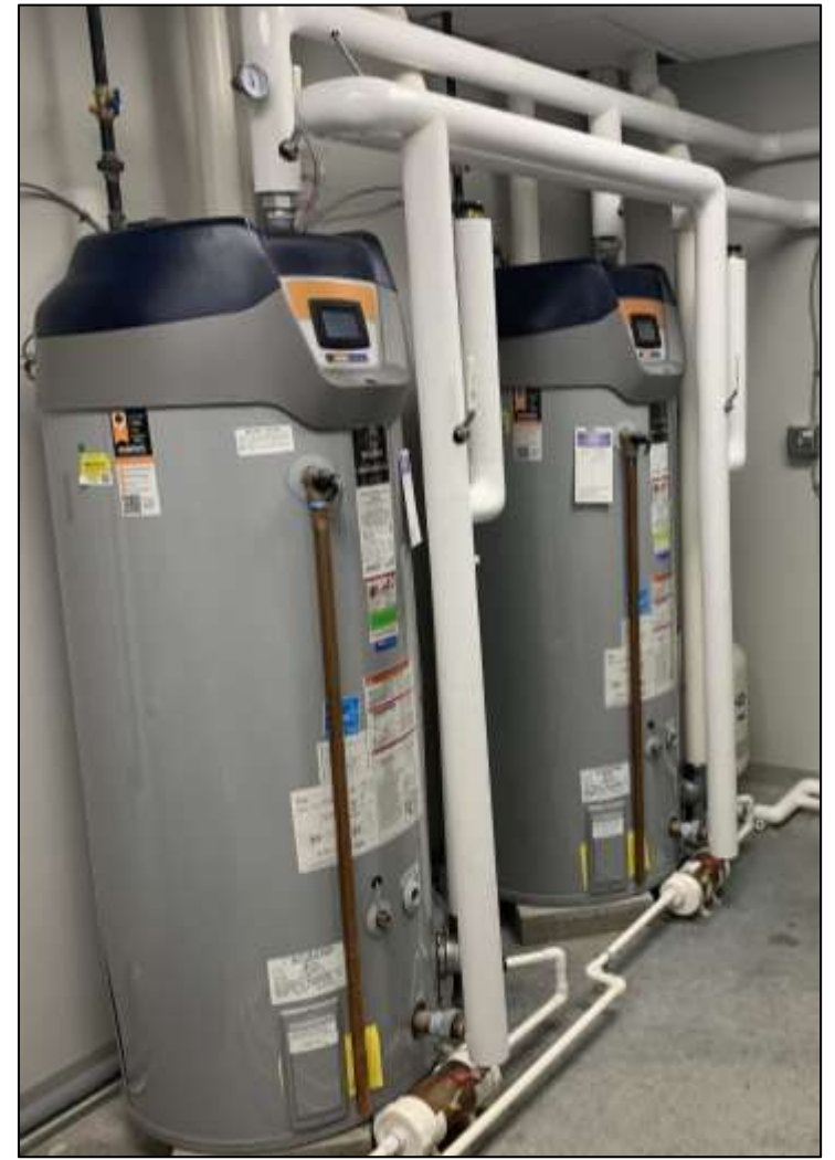
GAS DHW BOILERS
