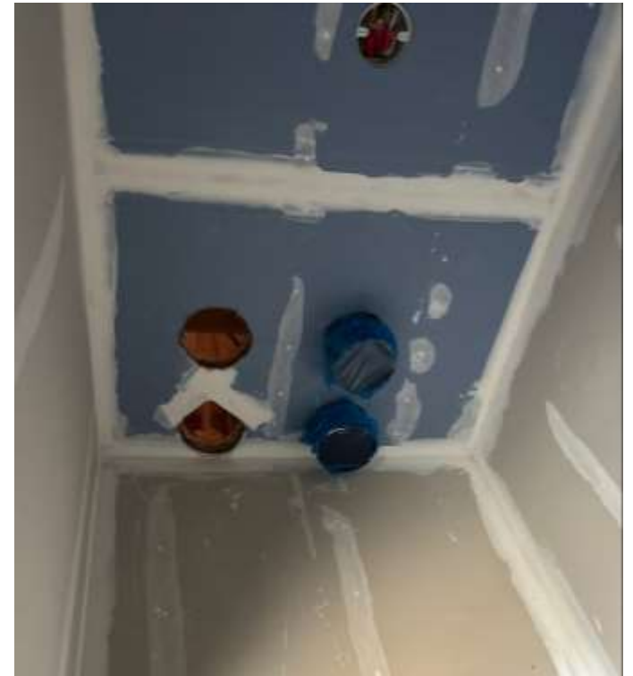
Limit attic penetrations
