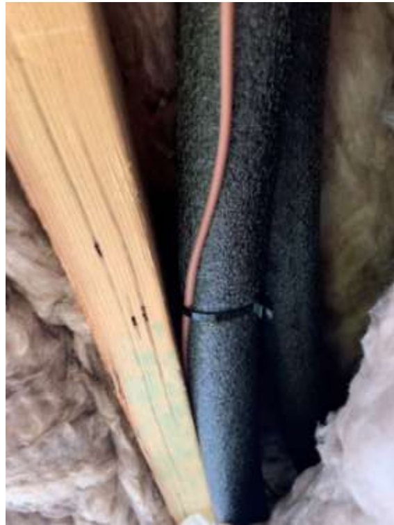
No pipes in exterior walls
